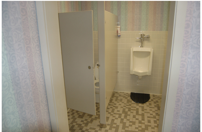
Non-Compliant Inaccessible Bathrooms
