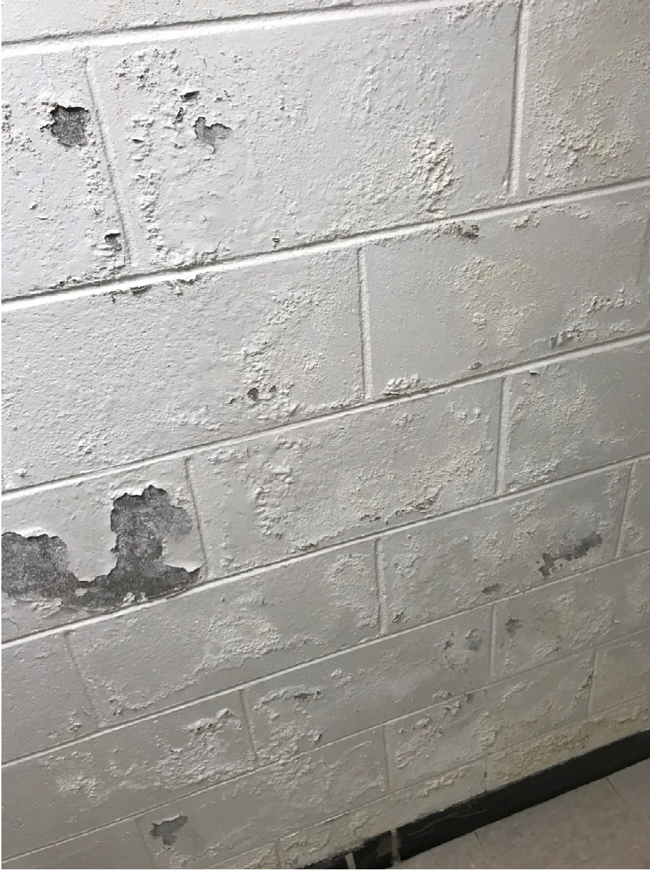
Picture #4. Water intrusion
