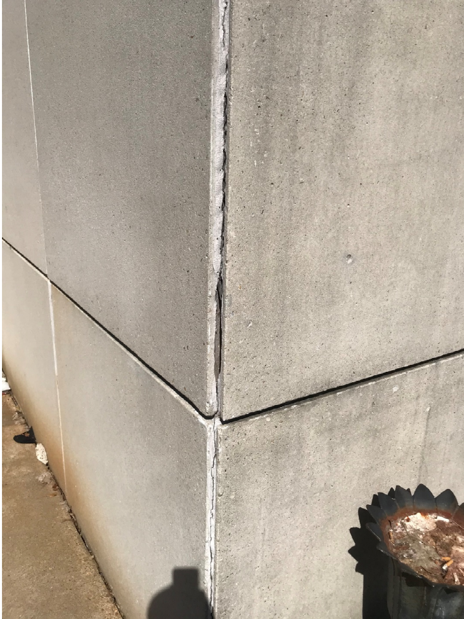
Picture #11. Precast joints appear to be failing
