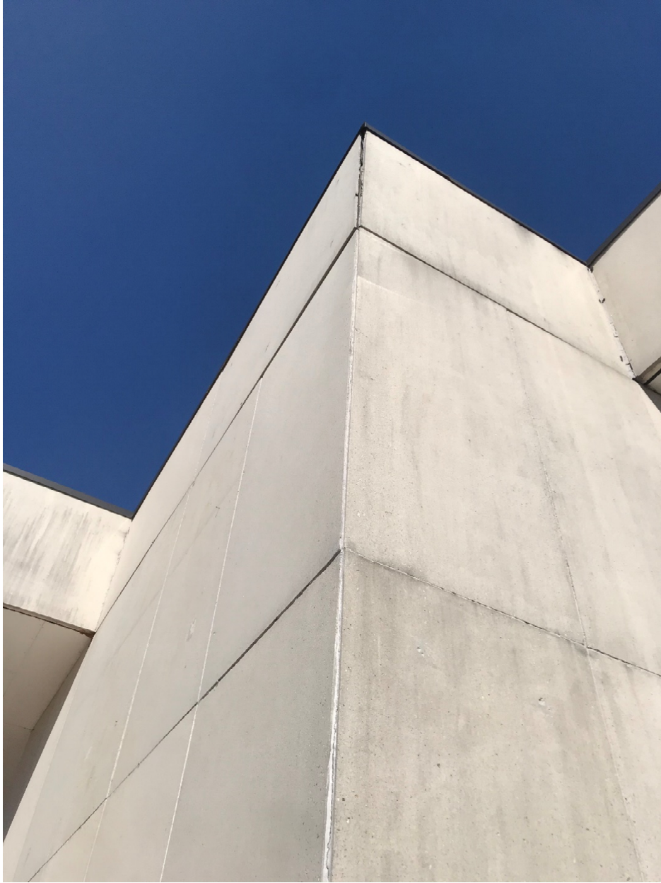
Picture #9. Precast attachment appear to be failing
