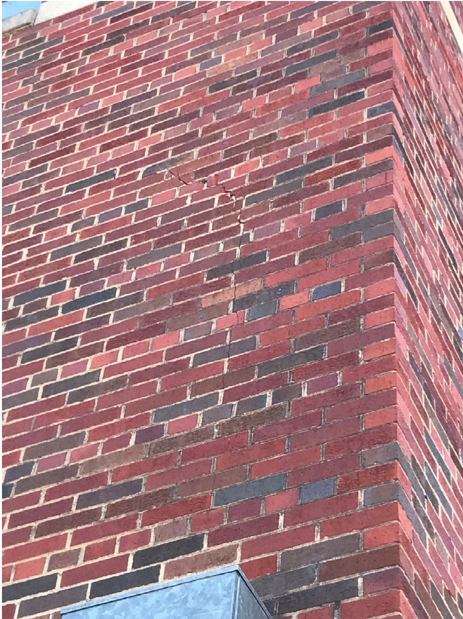
Picture #16. Crack in exterior brick
