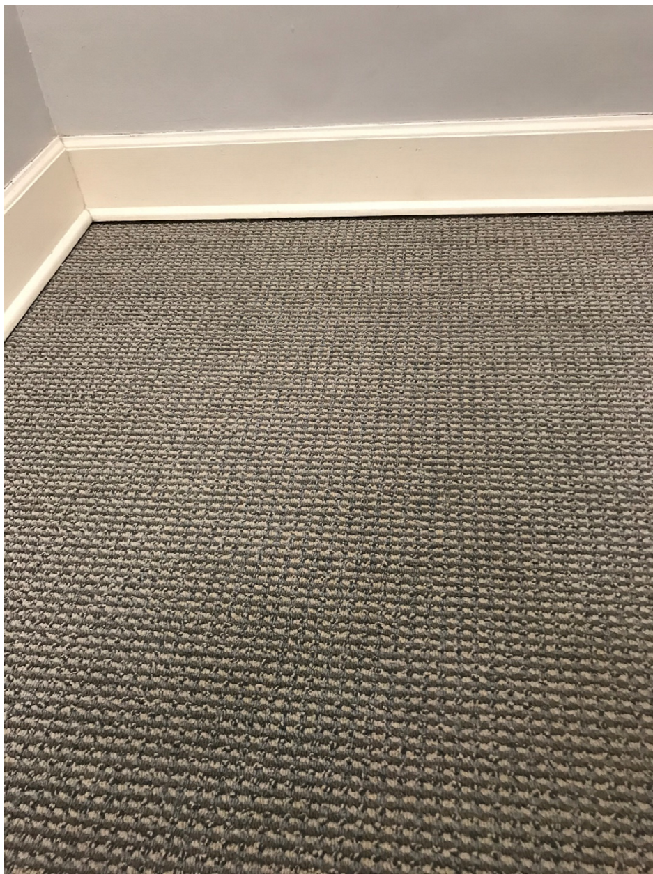
Picture #5. Are where floor appeared to sag
