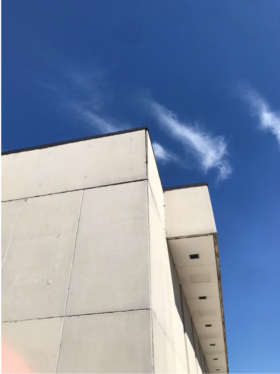
Picture #10. Precast pulling away from building
