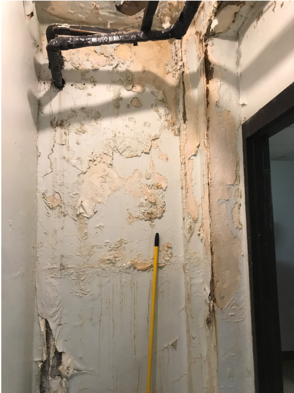
Picture #12. Water intrusion at police department
