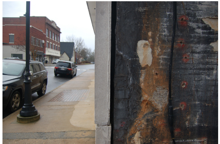
Unprotected Joint at Corner
