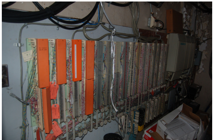
Existing Telephone/Low Voltage System
