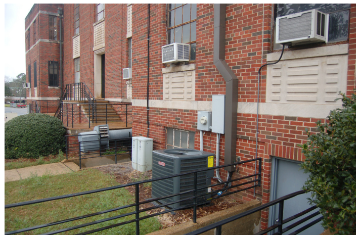
Diverse Mixture of Mechanical Systems
