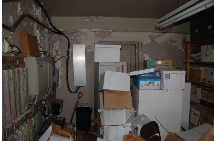
Access to Boiler Room where Hazardous Materials were Discovered.
