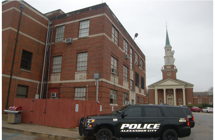
Uninsulated Steel Windows
