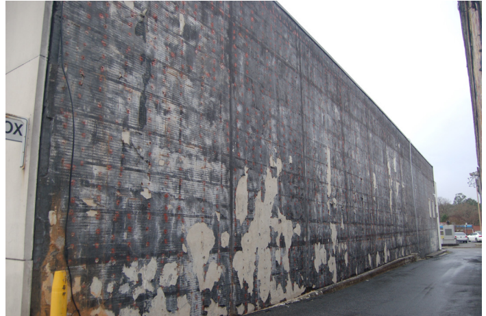
Exposed Wall Substrate where Stucco Removed
