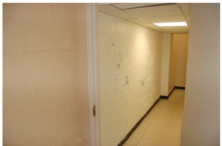
Water Intrusion at Lower Level
