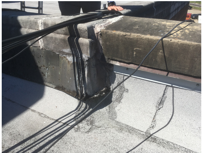
Area of Major Leak
