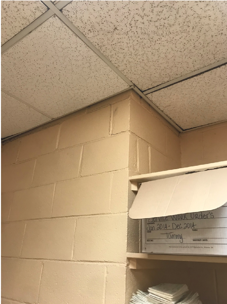
Picture #2. CMU cracks
