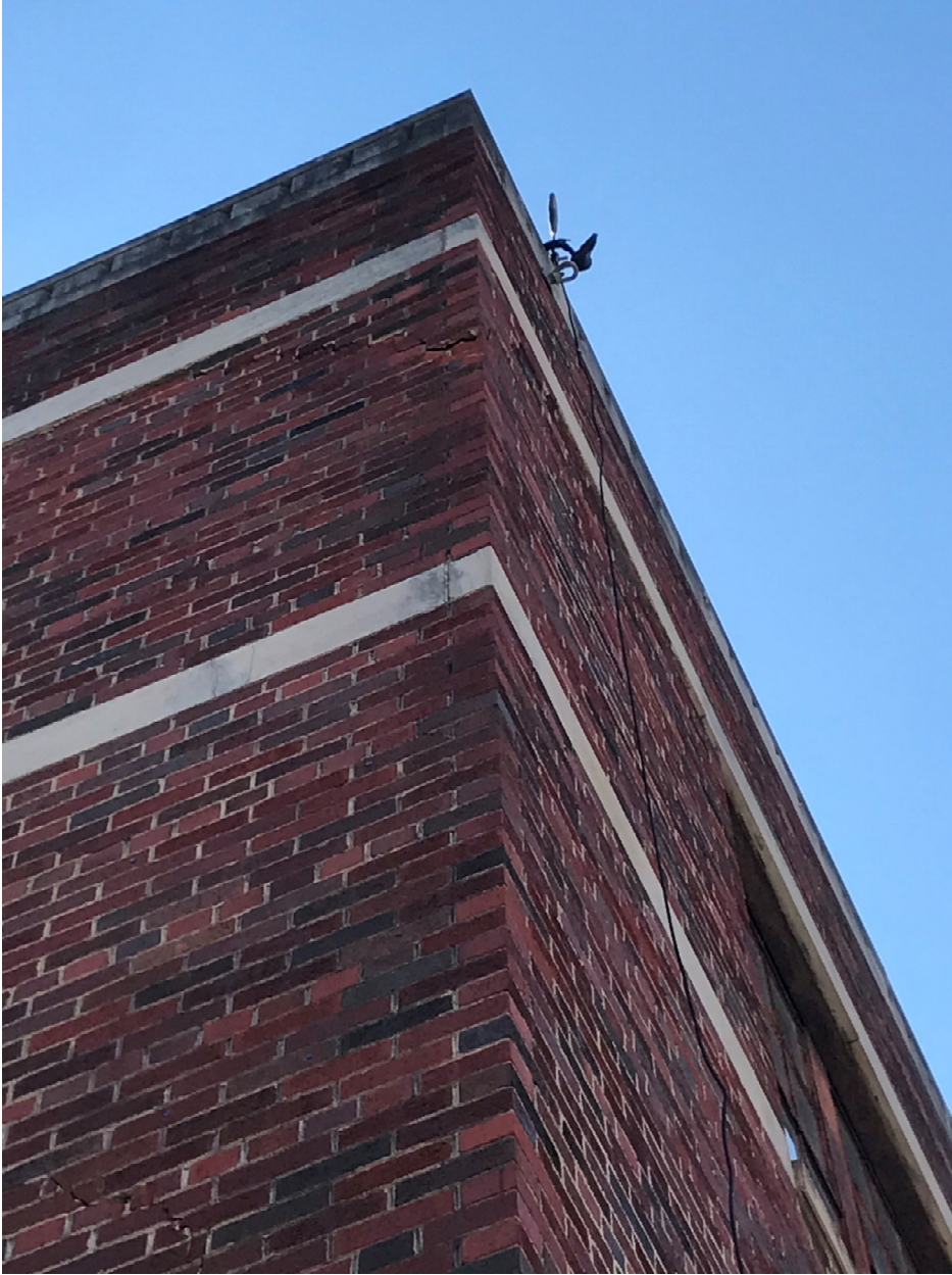
Picture #17. Crack in the exterior brick
