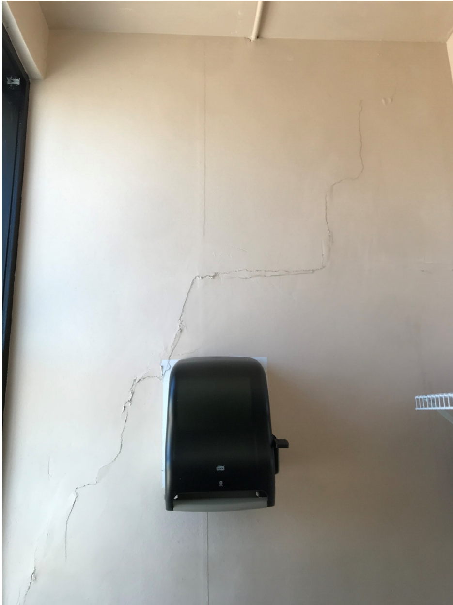
Picture #14. Crack in interior finish
