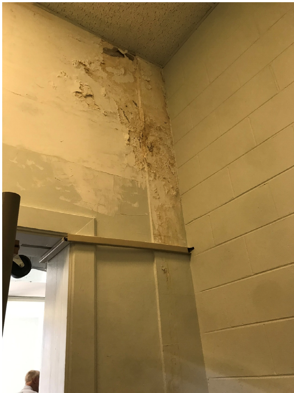
Picture #13. Water damage
