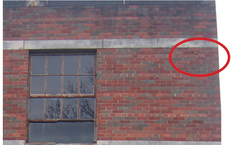
Cracks in Masonry
