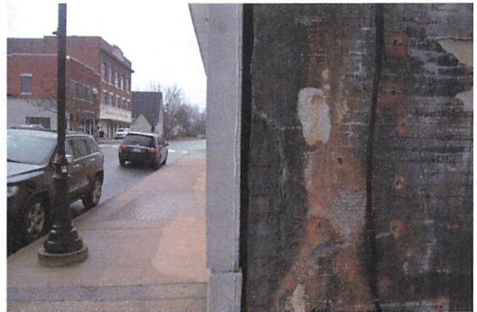
Unprotected Joint at Corner
