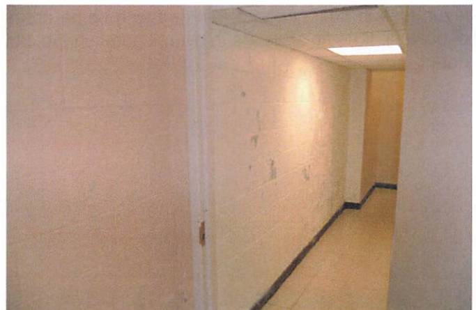
Water Intrusion at Lower Level
