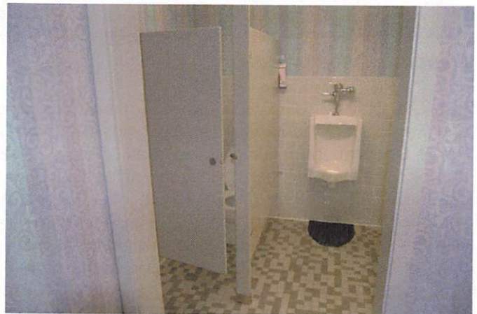
Non-Compliant Inaccessible Bathrooms
