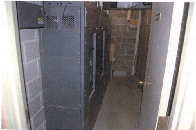
Existing Electrical Service
