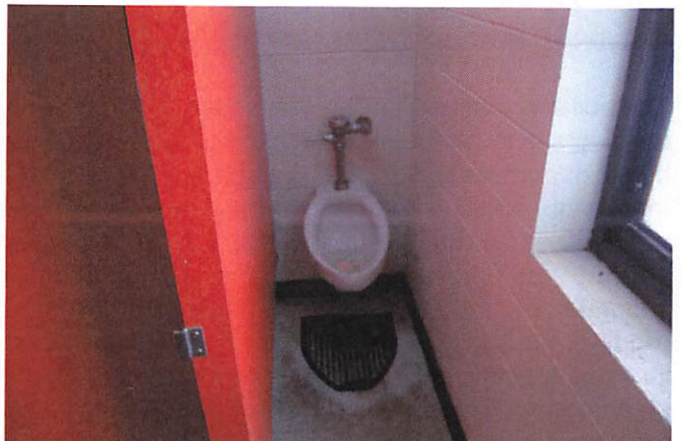
Current Non-Conforming Restroom
