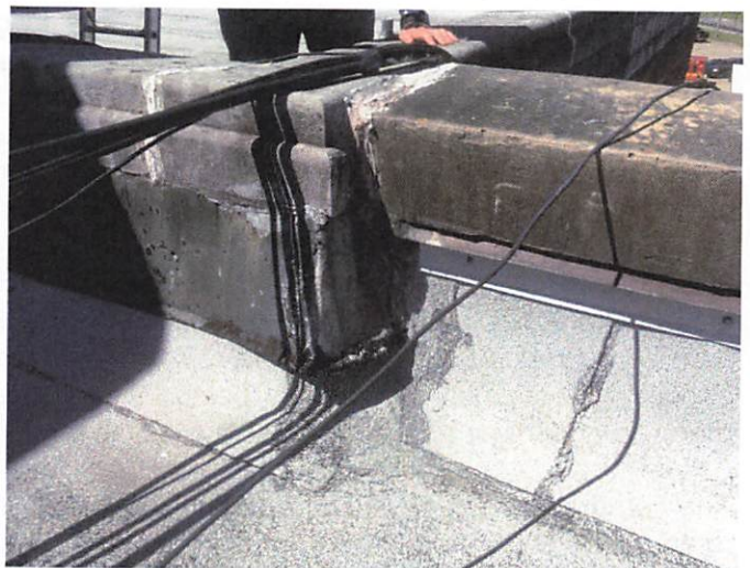
Area of Major Leak
