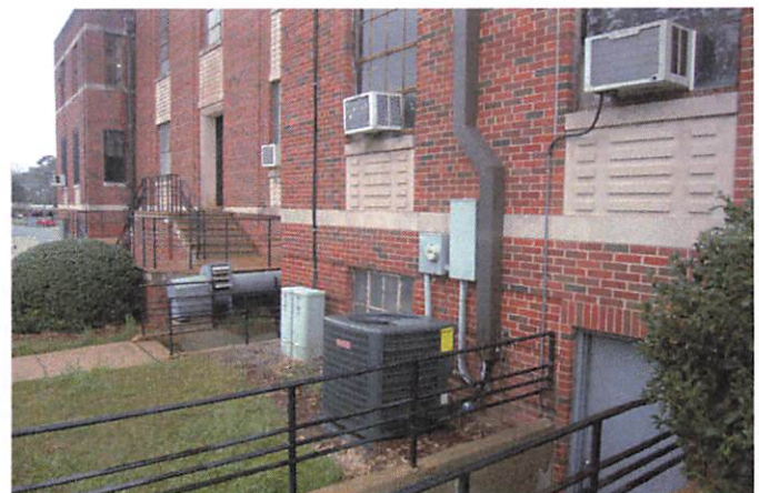
Diverse Mixture of Mechanical Systems
