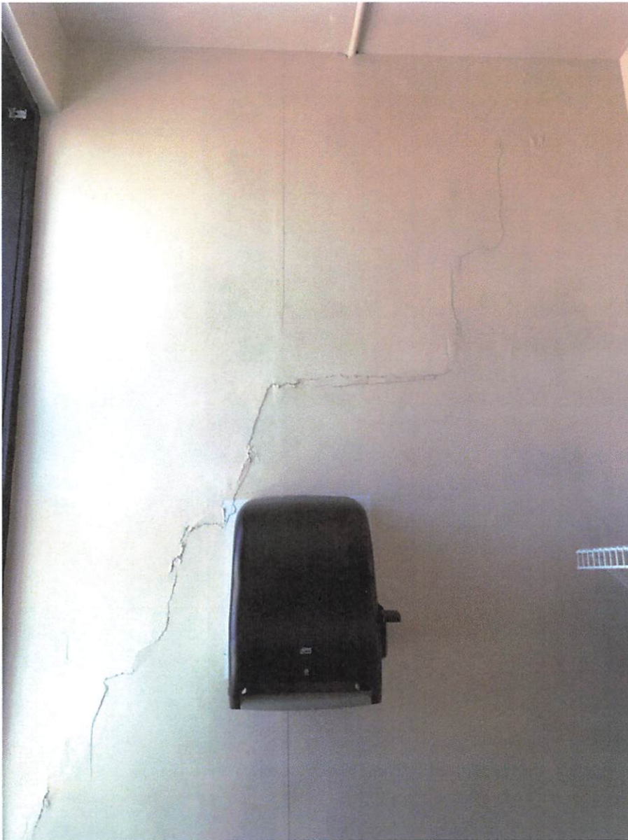
Picture #14. Crack in interior finish
