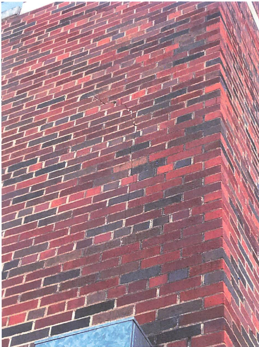
Picture #16. Crack in exterior brick
