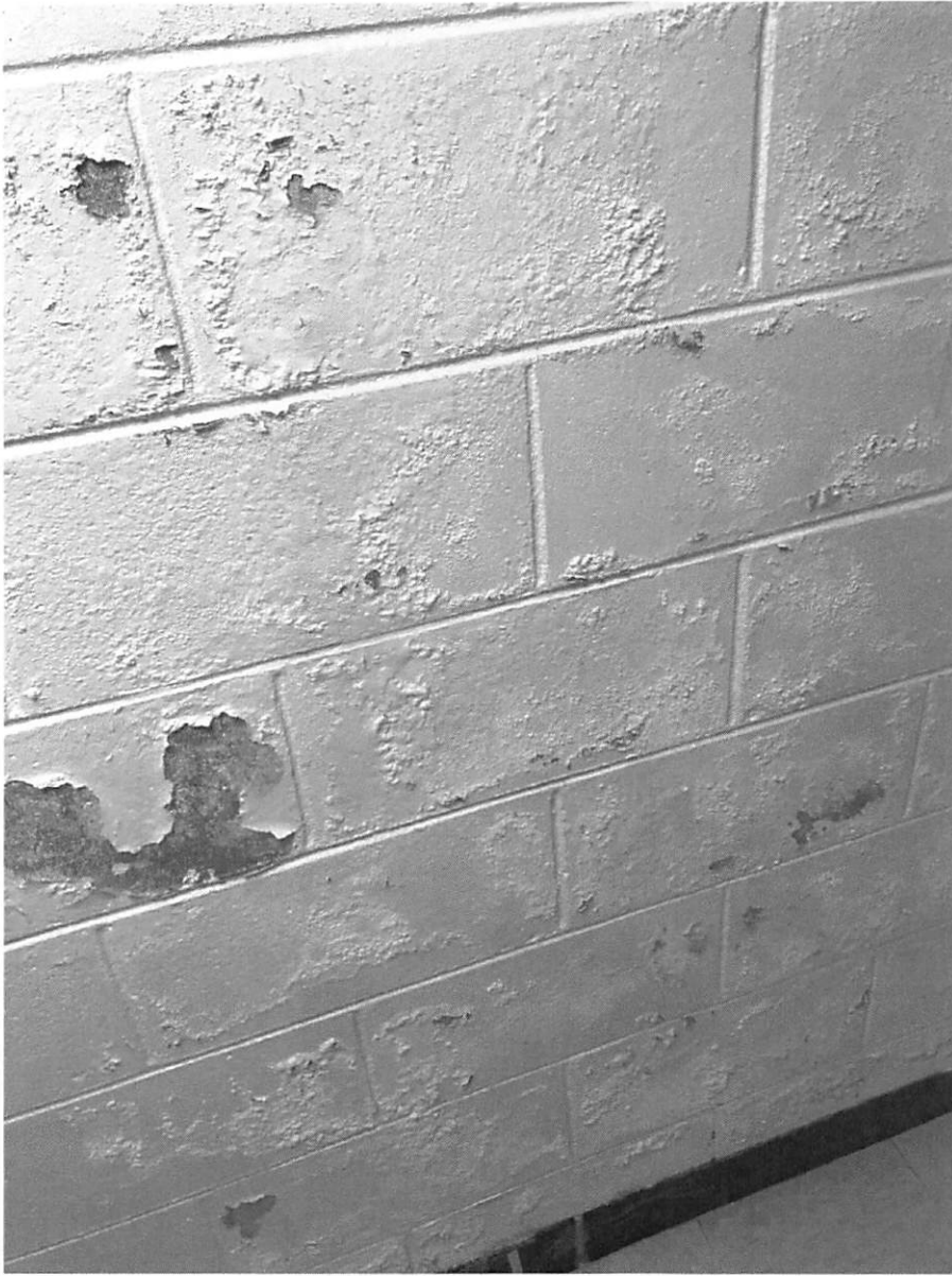
Picture #4. Water intrusion
