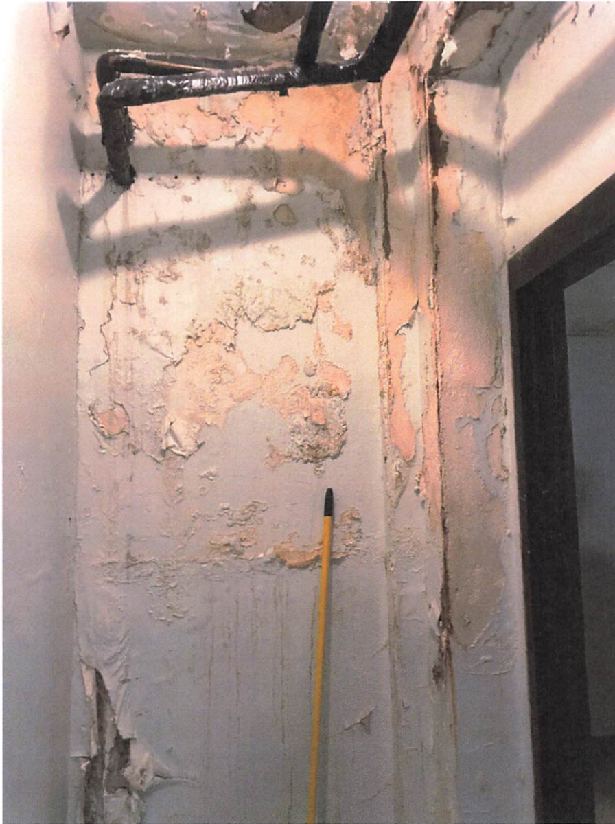
Picture #12. Water intrusion at police department
