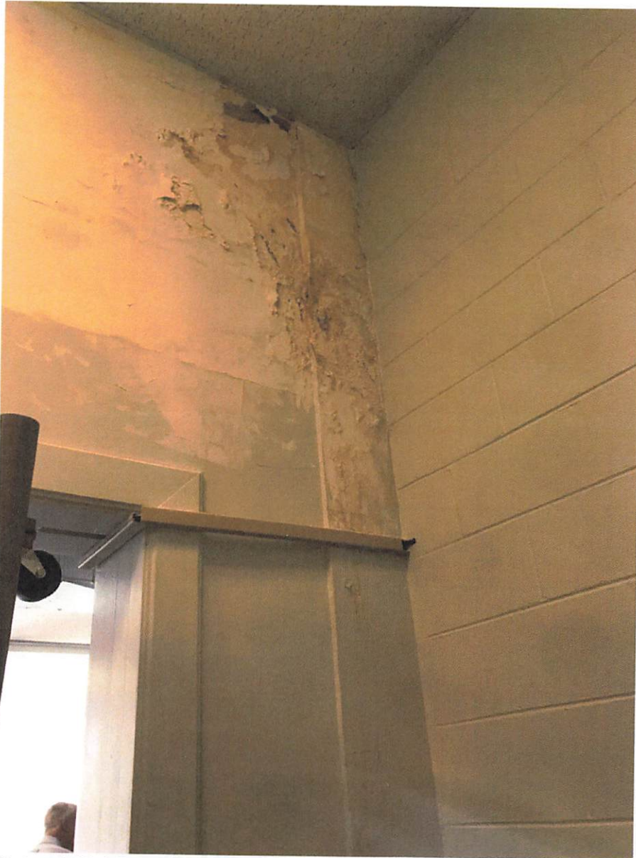
Picture #13. Water damage
