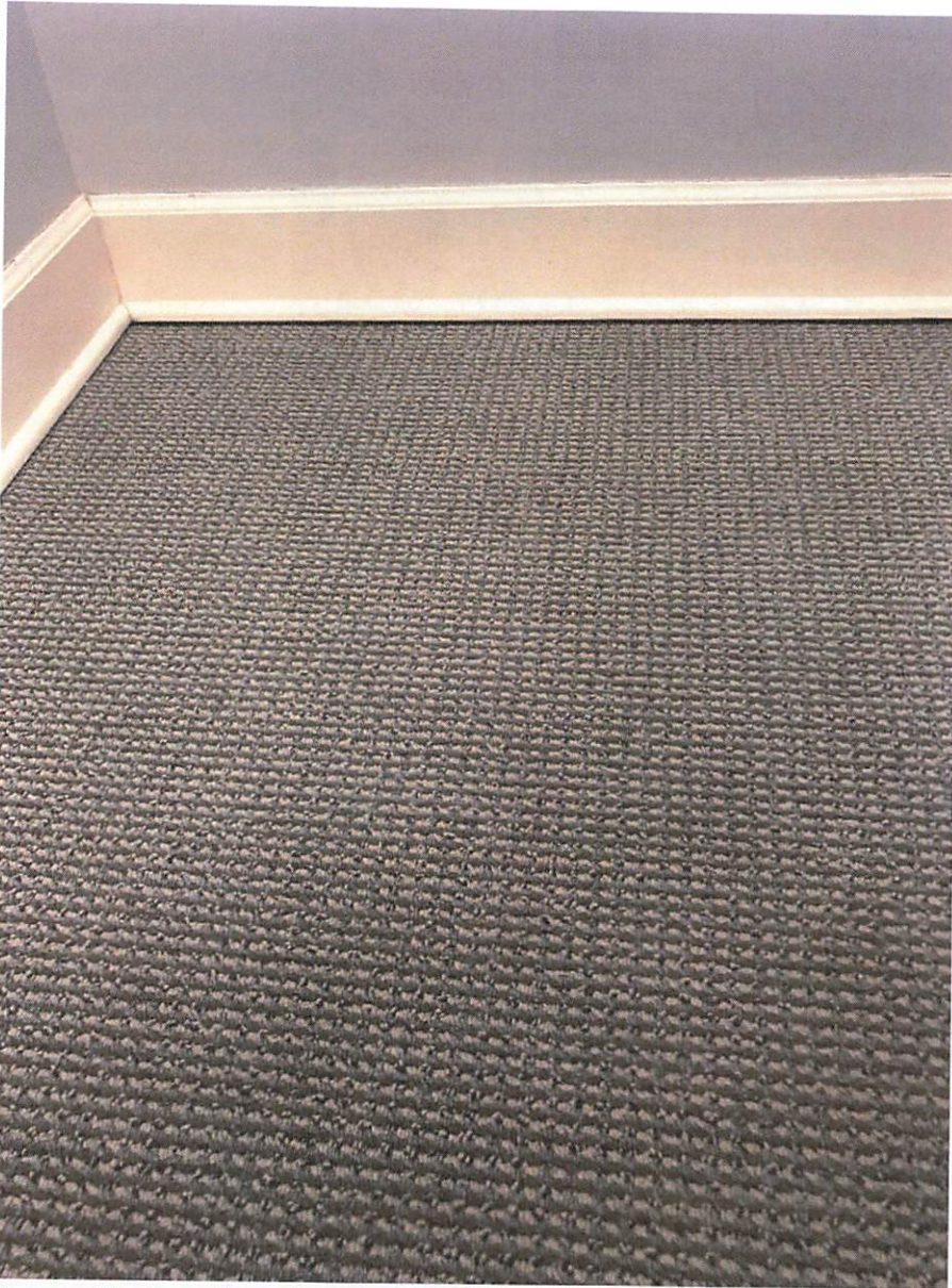
Picture #5. Are where floor appeared to sag
